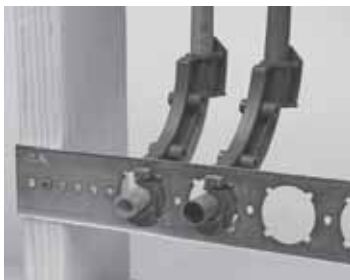
PEX Elbows installed in PipeSecure Bracket (P-1064)
